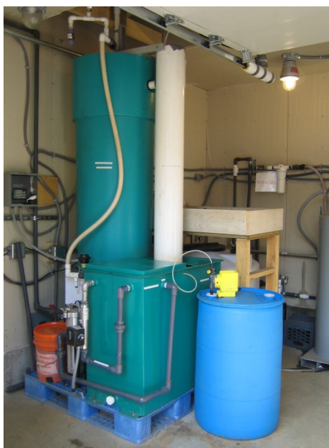
Figure 3. Small Bio-500 Located in New Hampshire.
