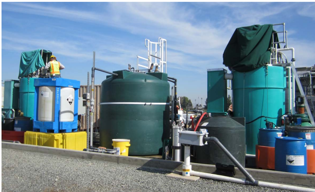
Figure 4. Bioreactor System in Norwalk, California showing an incoming process water surge tank (dark green), bioreactors (light green), HCl storage tank (white), and Nutrient and MTBE feed drums (blue).
