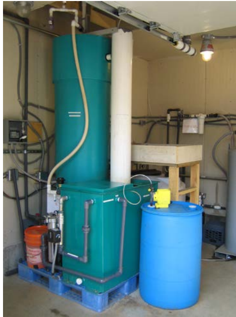
Figure 3. Small Bio-500 Located in New Hampshire.
