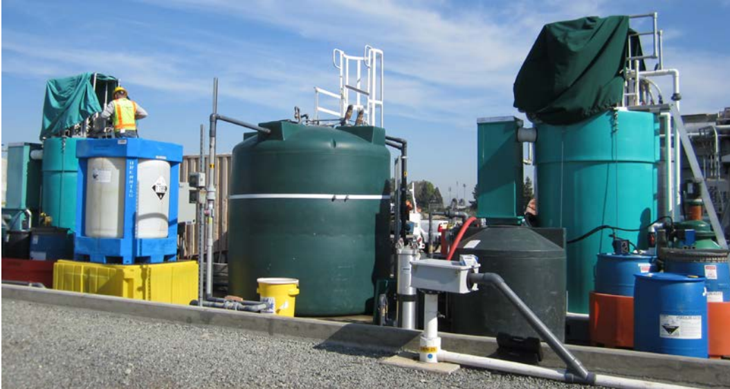
Figure 4. Bioreactor System in Norwalk, California showing an incoming process water surge tank (dark green), bioreactors (light green), HCl storage tank (white), and Nutrient and MTBE feed drums (blue).
