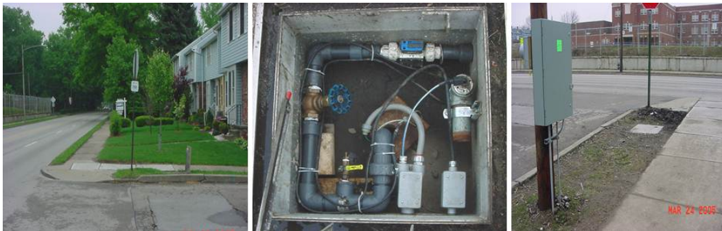
Figure 13. Installed MTBE Cut-off Pumping Well System - As-Built Photographs.
