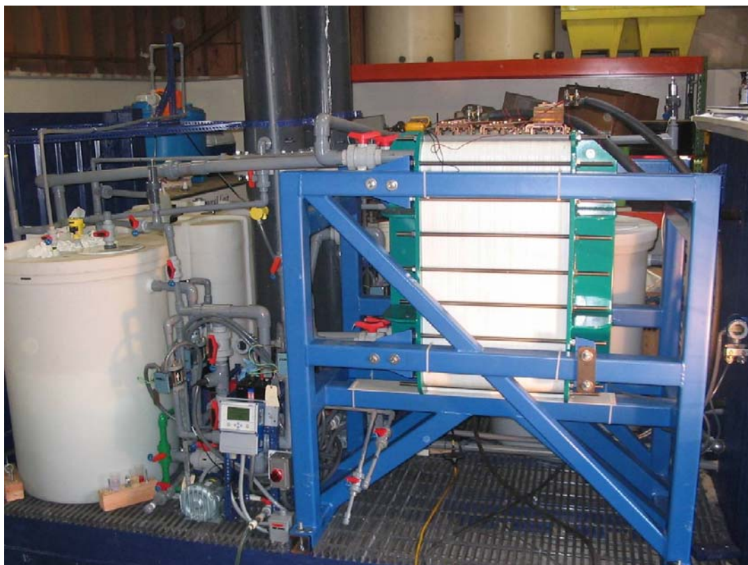
Figure 6. Electrochemical destruction unit for regenerant recycle
