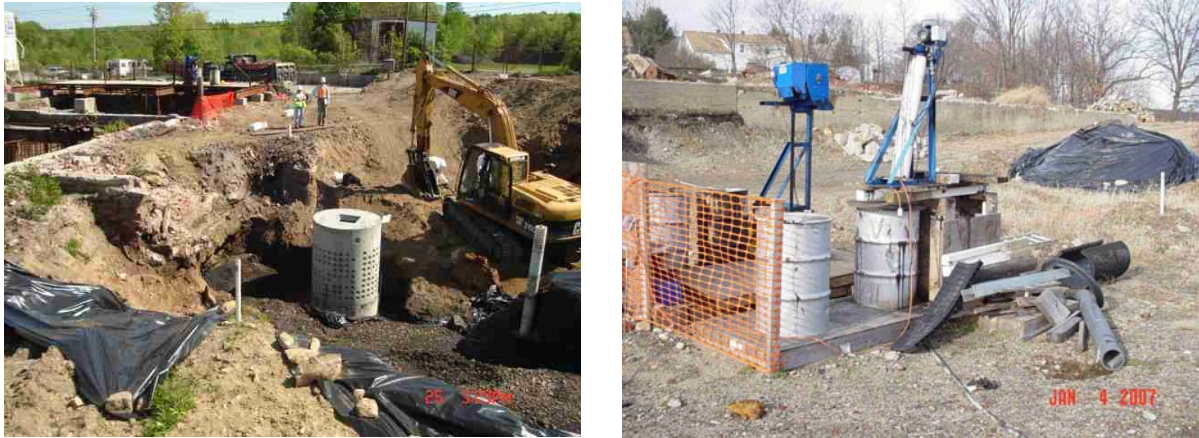
Figure 39(left). Installation of one of two recovery wells using perforated leaching basin sections.; Figure 40(right). Recovery wells fitted with belt skimmers.
