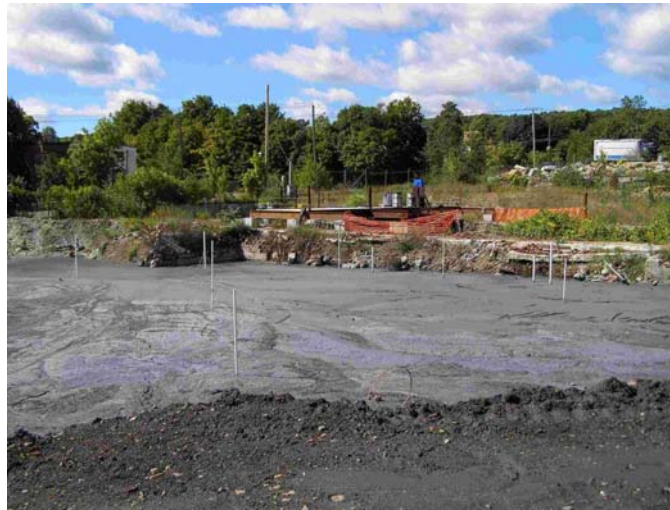
Figure 33. Application of flowable fill in front foundation area in conjunction with SVE piping, monitoring wells and injection points.
