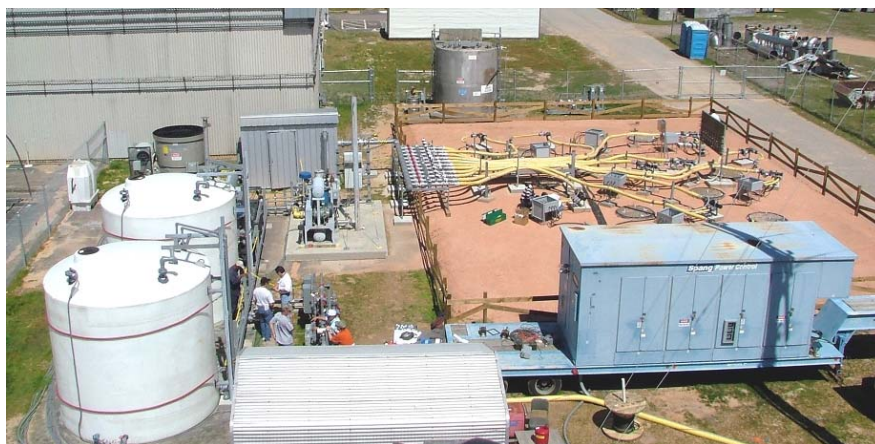
Figure 5. The ERH installation looking east. The electrode array is at top right, the electrical power supply is in the right foreground, the hut housing the control equipment is in the center foreground and the condensate tanks in the left foreground.
