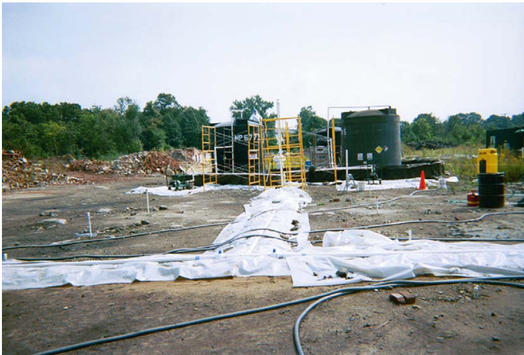
Figure 24. Permanganate Mixing Tanks and Distribution Manifold.
