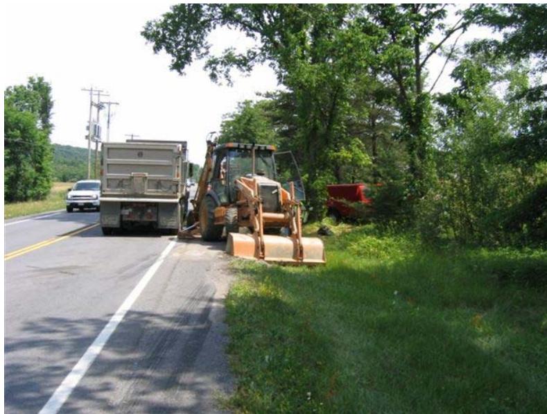
Figure 3. Accident site showing the asphalted road affected by spill.
