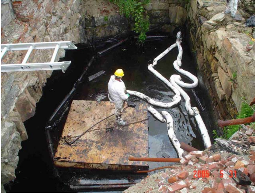
Figure 34. Oil absorbent boom change out in canal near tailraces
