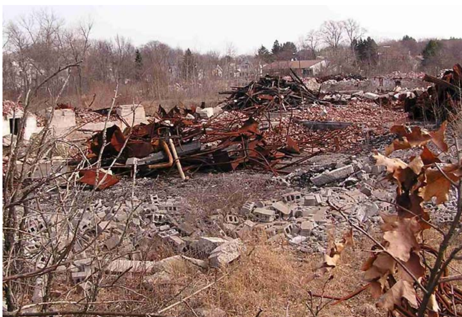
Figure 29. Debris piles at Fisherville Mill before remediation
