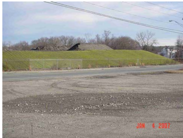
Figure 41. View of the site to the northeast across Main Street following application of flowable fill and re-use of offsite soil.
